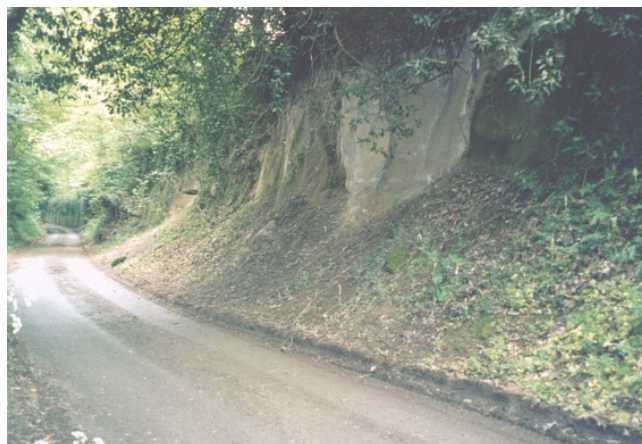
Photograph 2: Hartmoor Road, looking back towards the supporting wall, showing bank slippage
